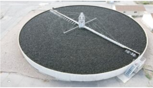
Trickling Filter (TF) 2
