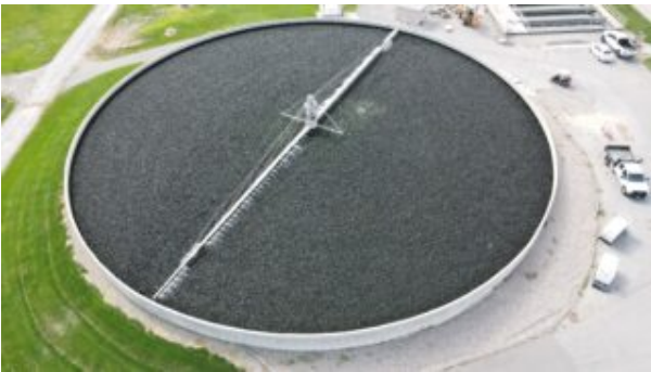
Trickling Filter (TF) 1
