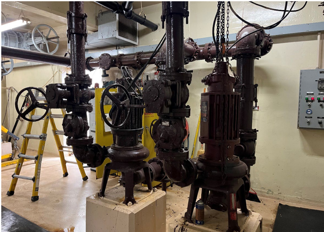
Figure 25: Second Stage Trickling Filter Pump Station
