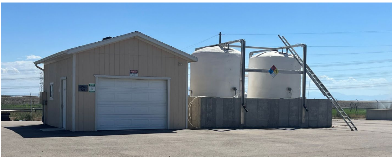
Figure 33: Sodium Hypochlorite Holding Tanks for Disinfection
