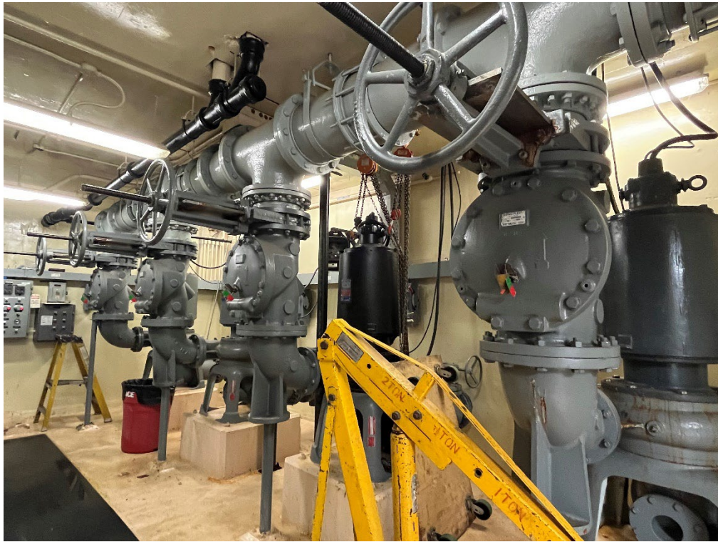
Figure 21: TF Sewage Pumps
