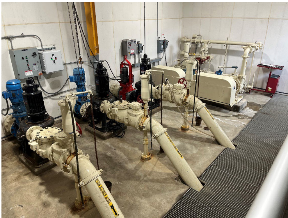
Figure 12: RAS and WAS Pumps for North and South Clarifiers
