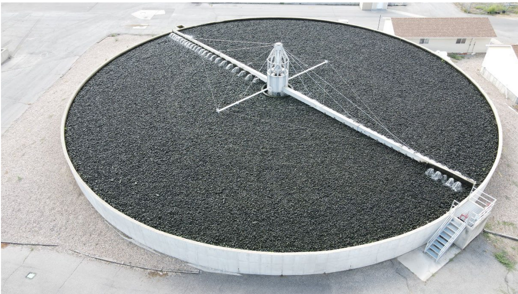
Figure 24: 2 nd Stage Trickling Filter
