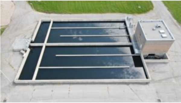
OD Chlorination Basin
