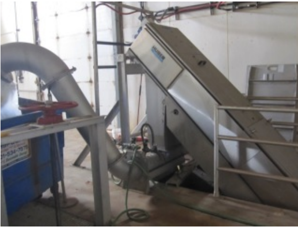
Screening Equipment Headworks
