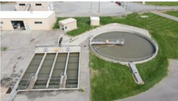
TF Primary Clarifiers
