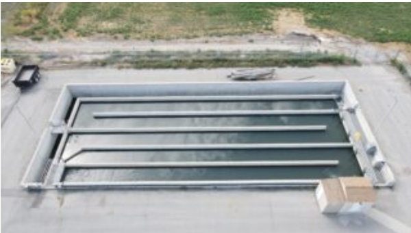
TF Chlorination Basin
