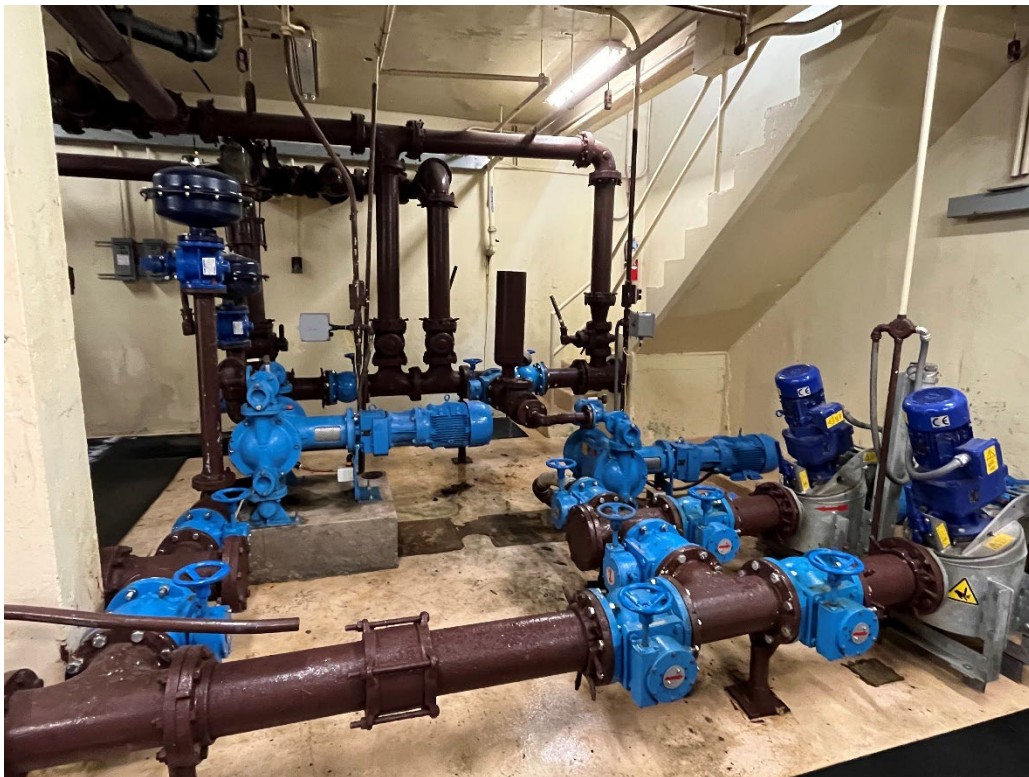
Figure 22: Sludge Pumps and Grinder
