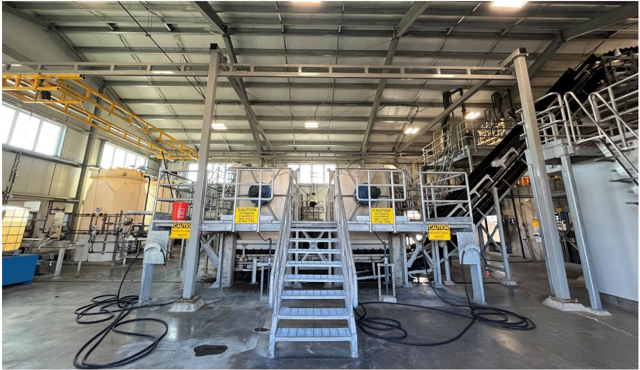
Figure 16: Inside Solids Handling for Oxidation Ditch Treatment Train
