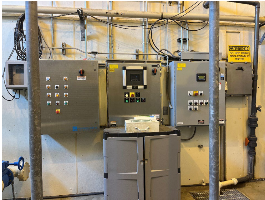
Figure 5: Headworks Electrical Panels
