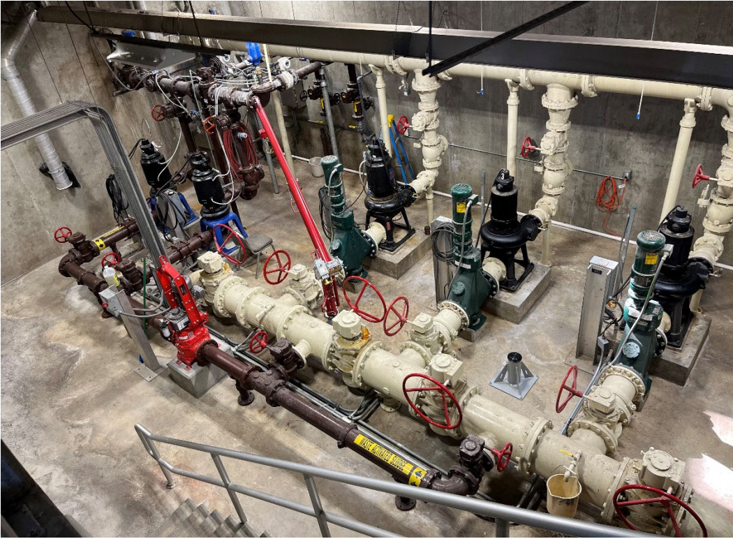
Figure 14: RAS and WAS Pumps for East and West Clarifiers
