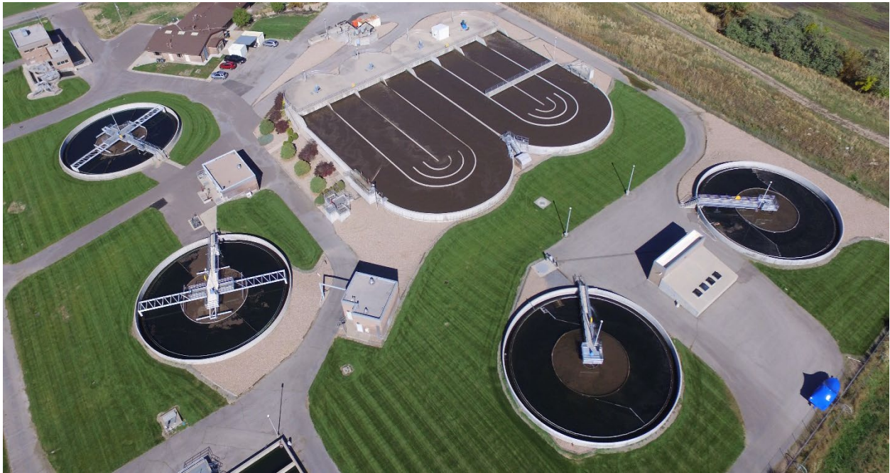
Figure 10: Oxidation Ditch Final Clarifiers
