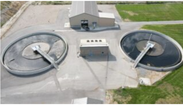
East and West Clarifiers
