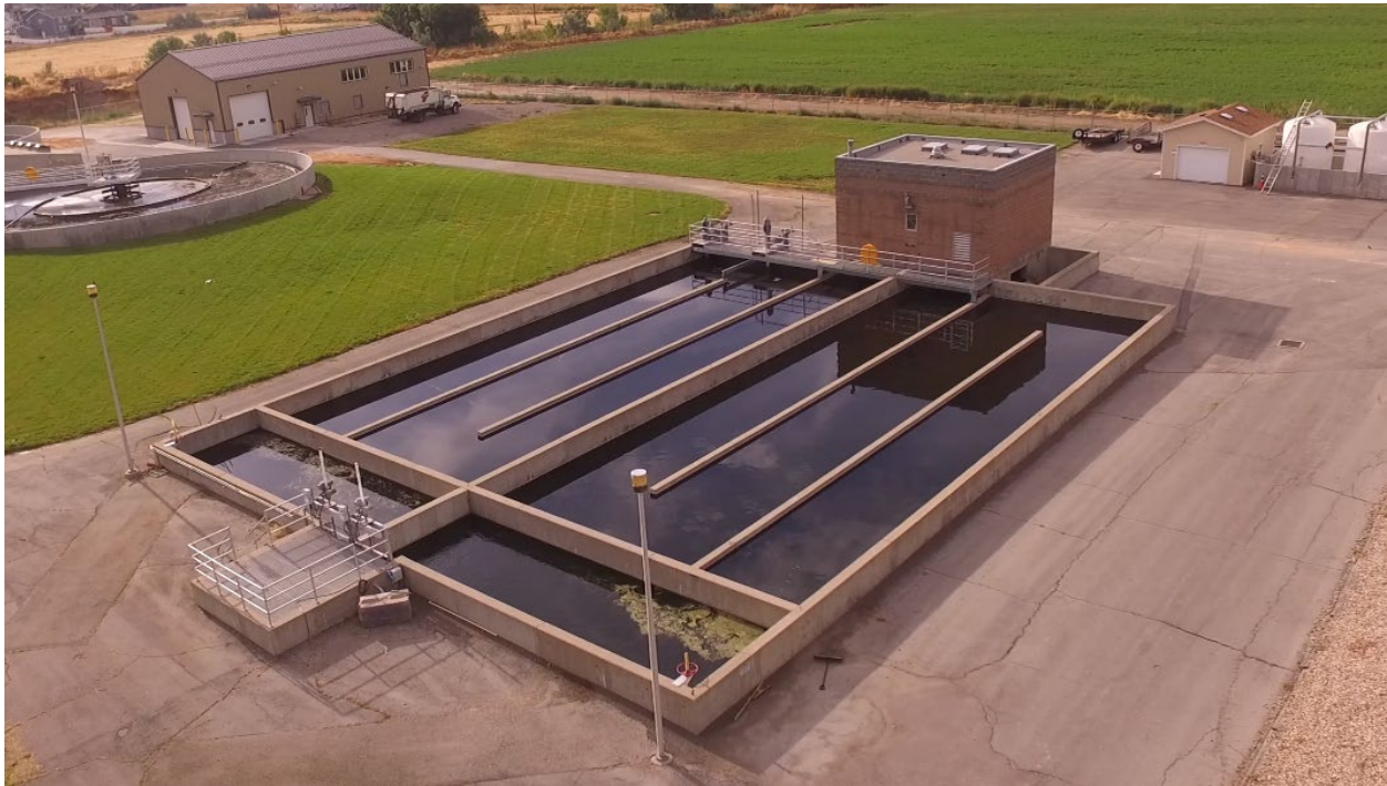
Figure 17: Chlorination Basin for Oxidation Treatment Train
