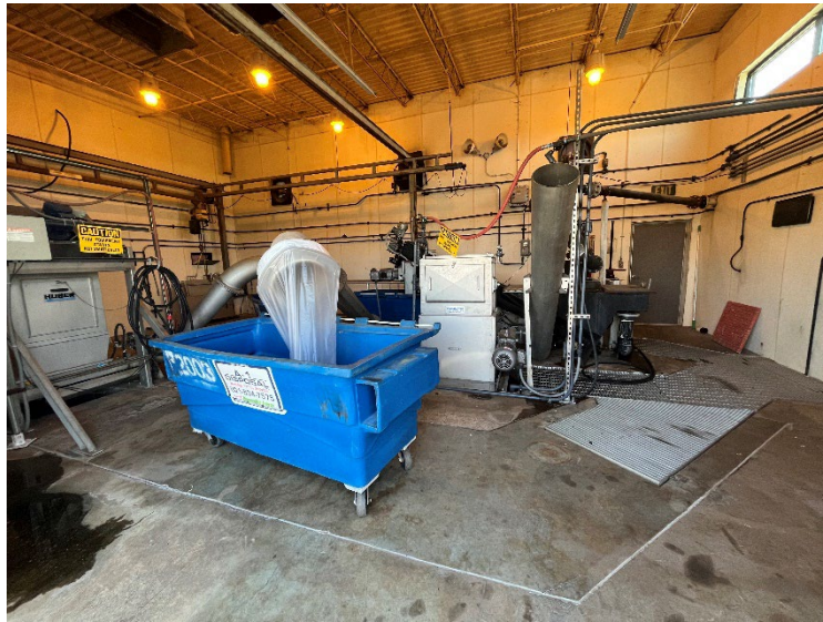
Figure 3: Headworks Screens/Compaction and Classifiers
